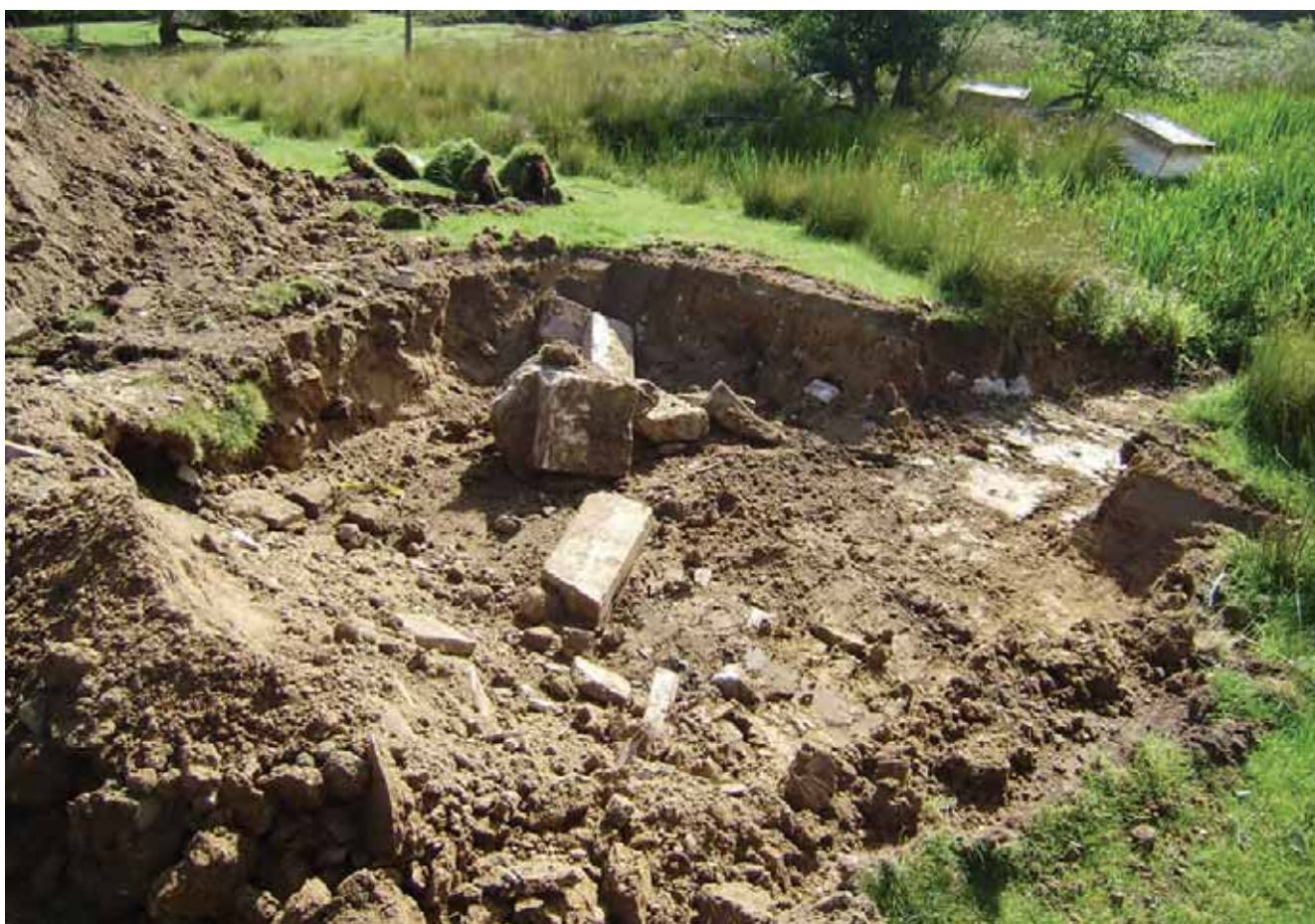
The basement of a hibernation site should be above the maximum pond level, so that rain water will drain to the pond instead of flooding the hibernation site.
