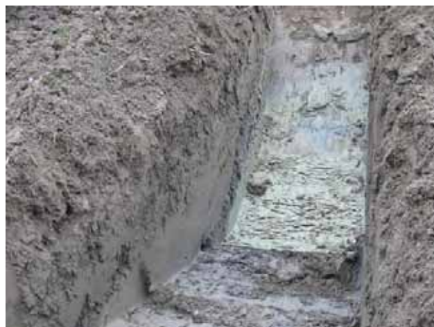
Blueish clay indicates an old waterbody. The sedimented or filled in top layers are removed to restore it.
