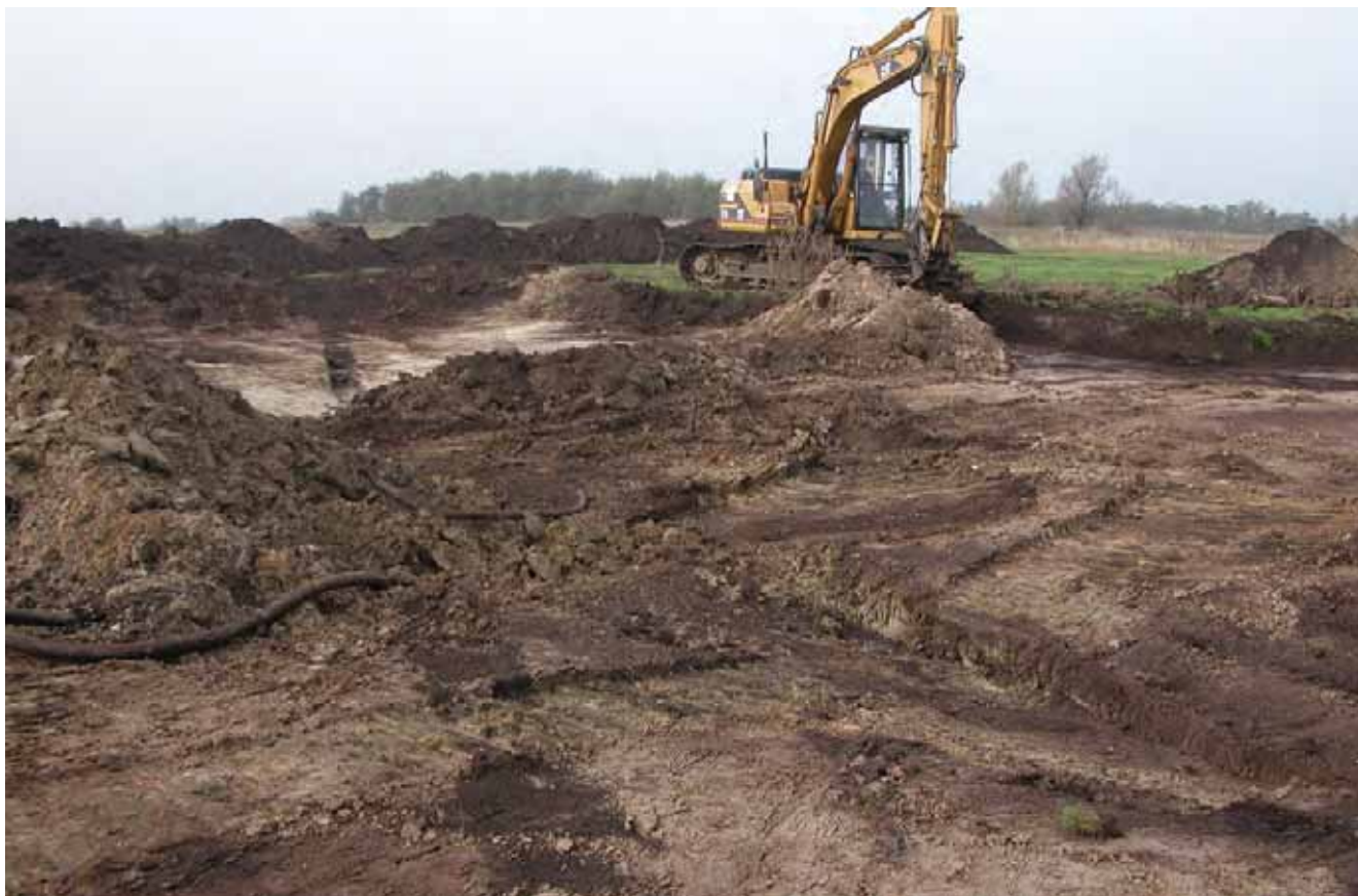
Drainages are found at almost all sites at different depths. In order to maintain water in the pond, these must be destroyed. The black line indicates the underlying drainage pipes.
